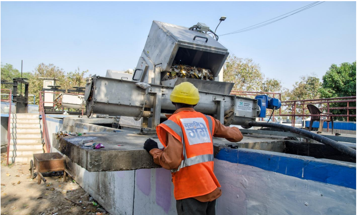
Figure 26: Worker at putting waste for processing at Naini Sewage treatment plant
